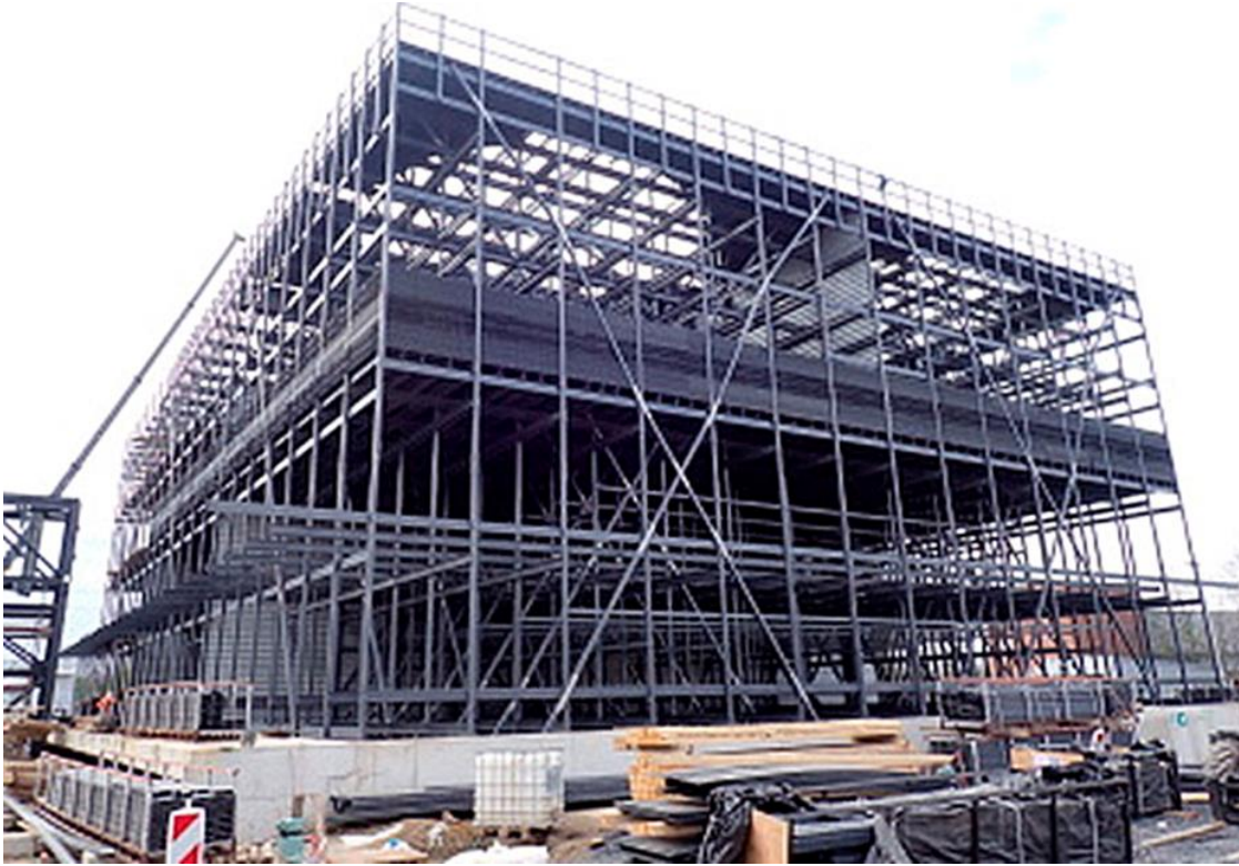
Fig.4-8: Fiber composites in building construction [Sorry. Originator not found in web]. The GFRP profiles of the cooling towers in the combined cycle power plant in Herne received approval on a case-by-case basis (Zustimmung im Einzelfall). In addition, the project-related type approval (Bauartgenehmigung) was granted for a cell cooling tower made of these GFRP profiles
