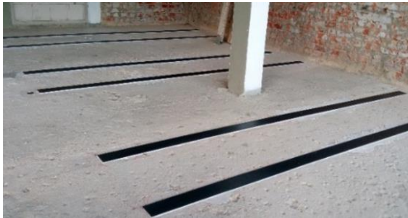
Fig.4-18 Rehabilitation of existing buildings: (up) Possibilities to strengthen by strip, pre-tensioned or slack. (down) Reinforcement of slabs because of increased moments by CFRP-lamellas, hydrostatic pressure from ground, applying External Reinforced Bonding ERB. Mineralbad "Berg", Stuttgart, 2018, [HPTL]. And for post-reinforcement of slab break-throughs to capture the local stress concentrations Refurbishment by reinforcement of Beam and slabs
