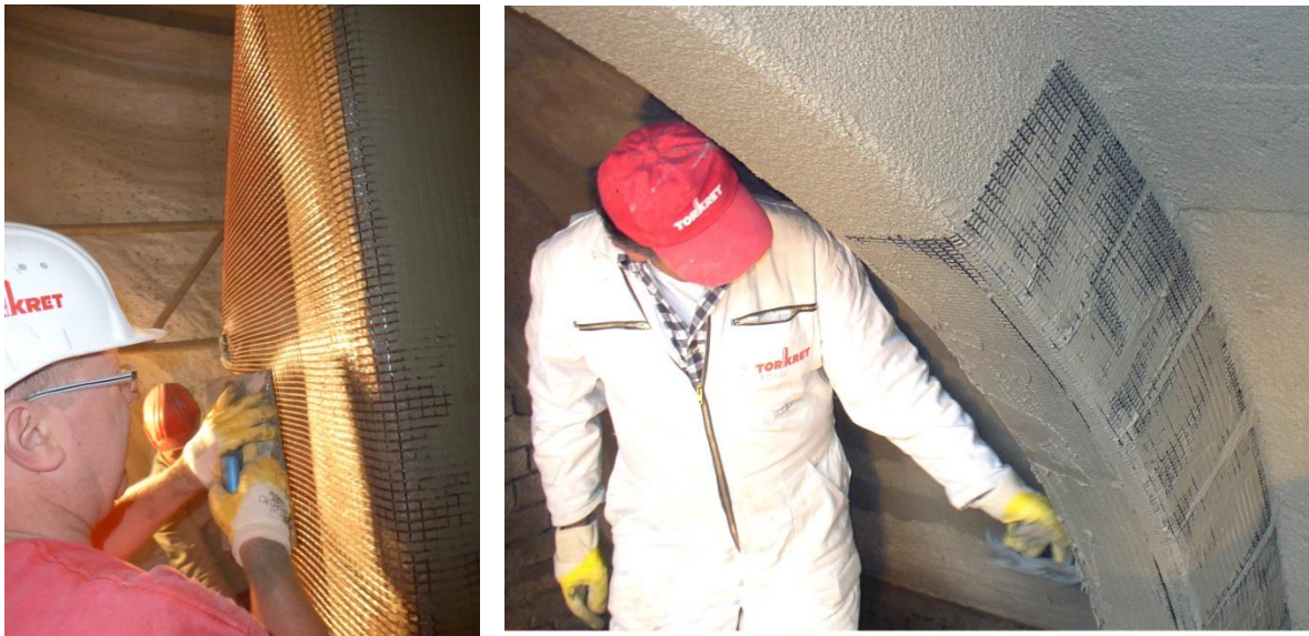
Fig.17: Verstärkungen in Carbonbeton /Retrofitting with Carbon Concrete [Torkret]. (links) Innenstützenverstärkung, Berlin; (rechts) Tonnengewölbeverstärkung, Finanzamt Zwickau. (left) Internal supporting pillar, Berlin; (right) Barrel vault reinforcement, tax office Zwickau
