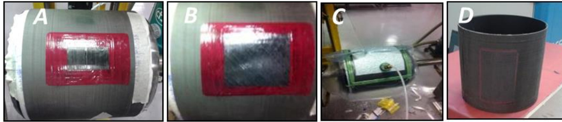
Figure 9. Hand lay-up of the repairing patch, vacuum bag and repaired scaled cylinder Skirt
