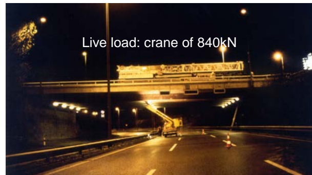
Figure 8. Ibach Bridge during loading test after application of externally bonded CFRP strips.
