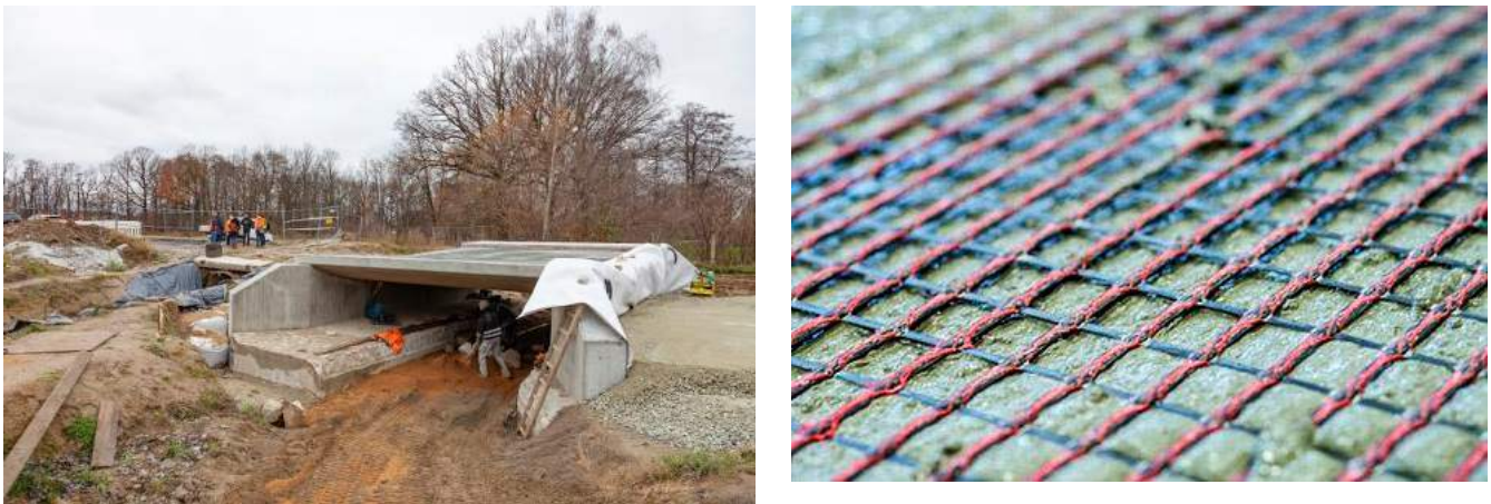
Fig.21-1: Bridge Wurschen, 2022: (left) Superstructure made exclusively of carbon concrete, shell construction. (right) Textile FRP mats in the super-structure) (Foto: Stefan Gröschel, IMB, TU Dresden)
